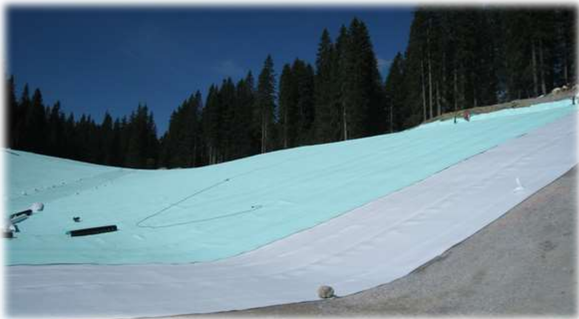
Figure 3: Membrane MAPEPLAN T WT on water reservoir
